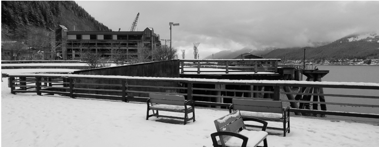
Figure 4: Photo showing the elevation difference between the southeast (Steamship Dock) and northwest (Wharf Mall) portions of the seawalk, photo from the northwest side.
