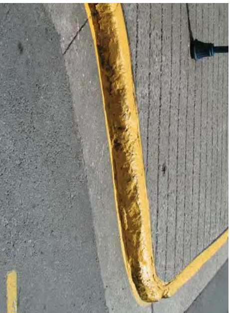
Curb and gutter throughout the project area and particularly at the curb-bulbs has been badly damaged by maintenance activities.
