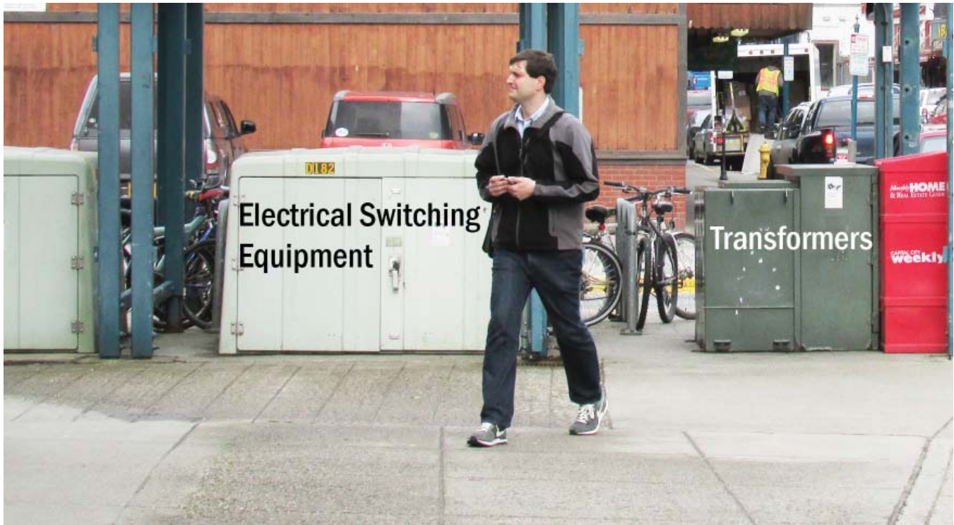
Electrical switching equipment and transformers near intersection of Ferry Way and South Franklin Street
