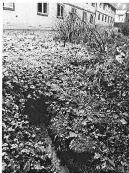
Figure 1: Existing Ditch (Right) and Location Where Groundwater Enters the Ditch (Left).
