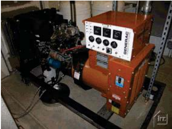
Back up power generation
