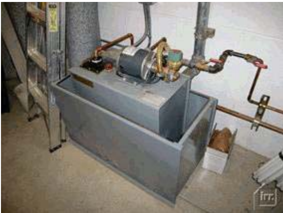
Day oil tank
