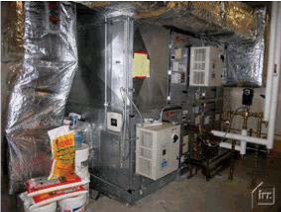
Dual air handler system
