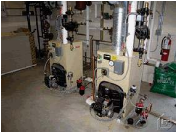
Dual boiler system
