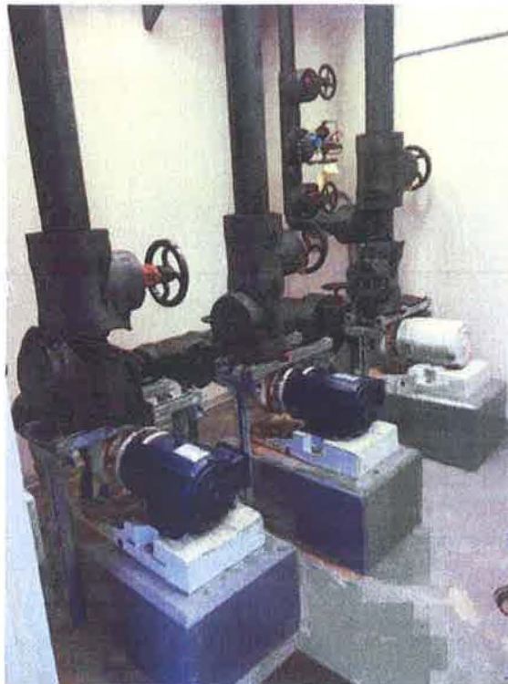
Mountainside Estates Pump Station
