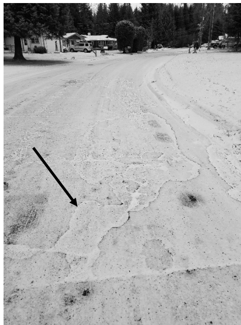
Left: Severe transverse cracks on Aspen Avenue near East Valley Court are packed with snow.
