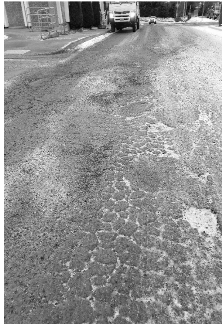
Left: Alligator cracking down the middle of Hospital Drive, approximately 500 feet from Old Glacier Highway.
