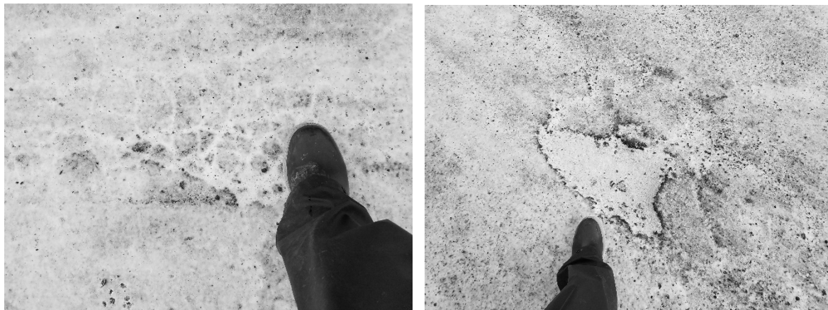
Left: Snow packed into severe alligator cracking. Right: Pothole resulting from severe alligator cracking. The women's size 8 boot is provided for context.
