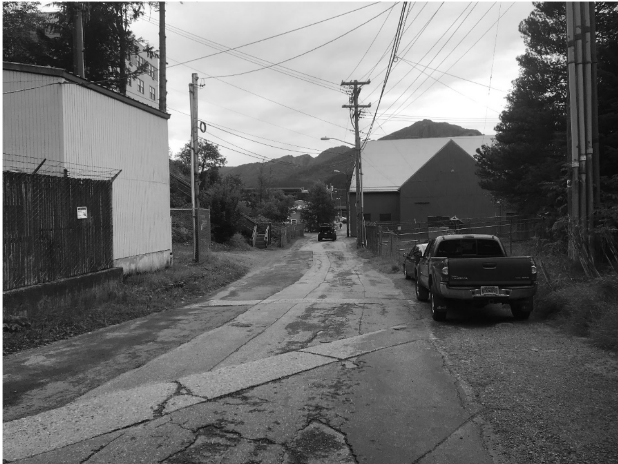
Capitol Avenue's current asphalt conditions. On the distant right an old style luminaire can be seen. Slide 6 of the Design Public Meeting deck.
