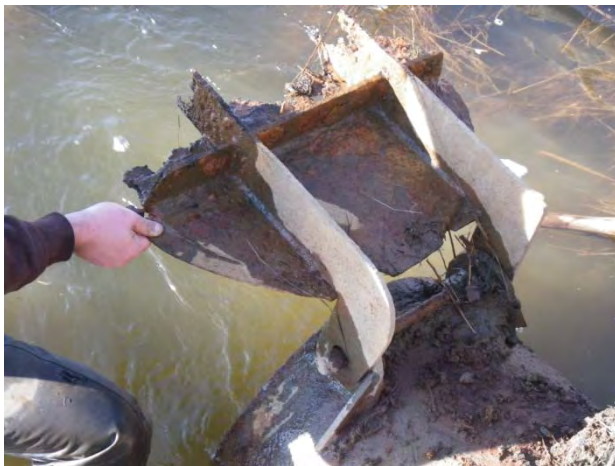
Figure 11. West berm failed culvert flap.
