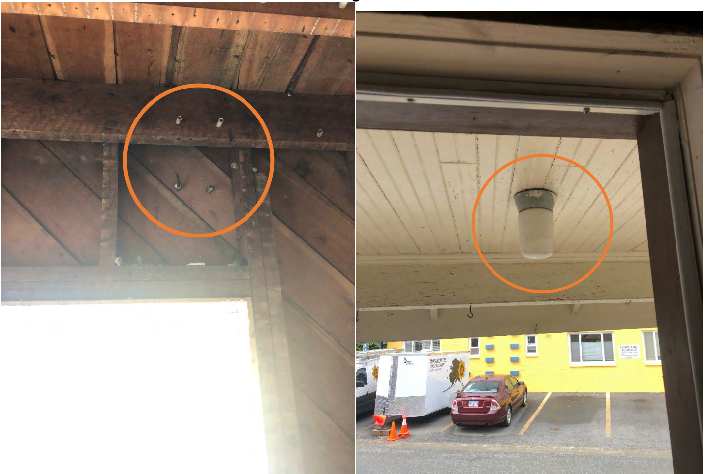
LEFT: Knob and tube wiring above the front door leading to shed entry lighting fixture.
