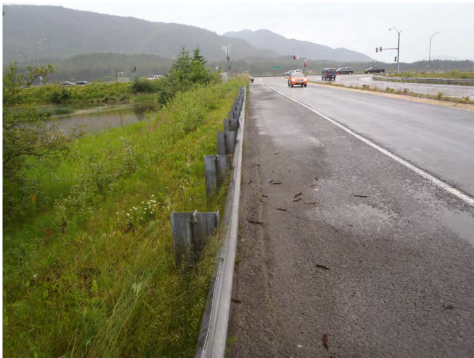
Figure 5 - Flattened Guardrail near Station 90+50 Adjacent to the North East Bound Lane, Looking South West
