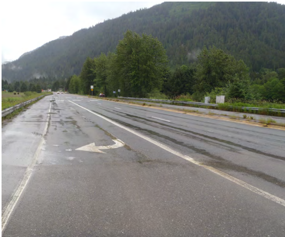
Figure 3 - Right-hand Turning Lane and Pavement Joint Looking North East
