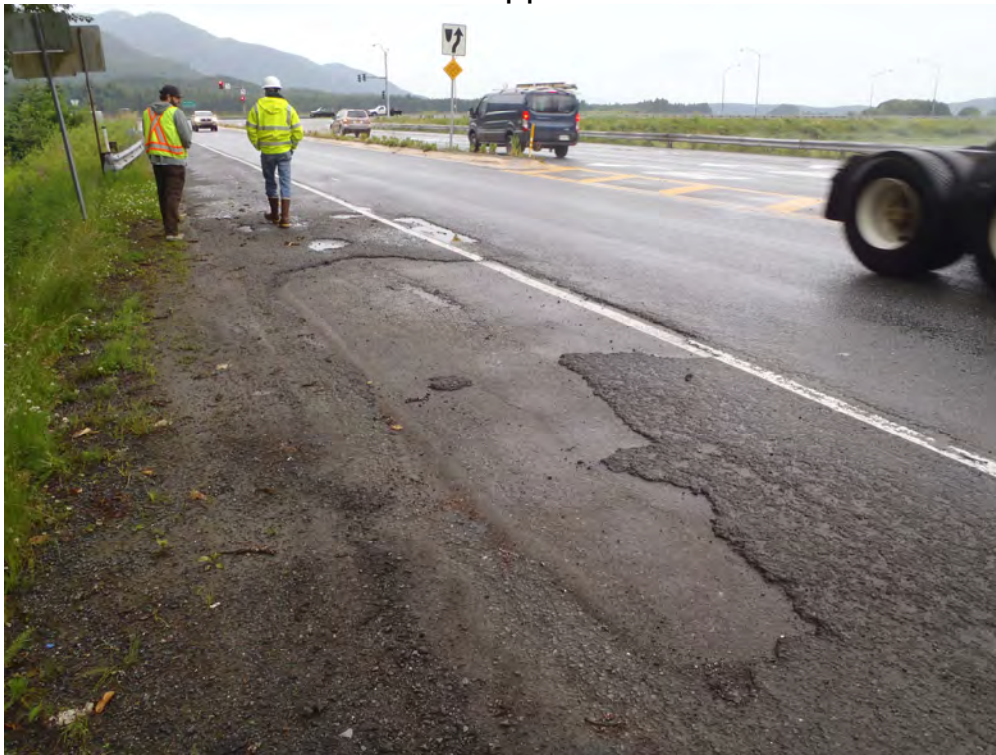
Figure 4 – North East Bound Shoulder Conditions near Station 92+50
