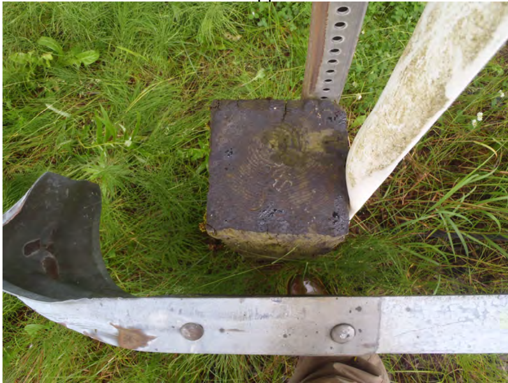
Figure 6 - Missing End Terminal Connection on the Southern Guardrail near Station 91+20
