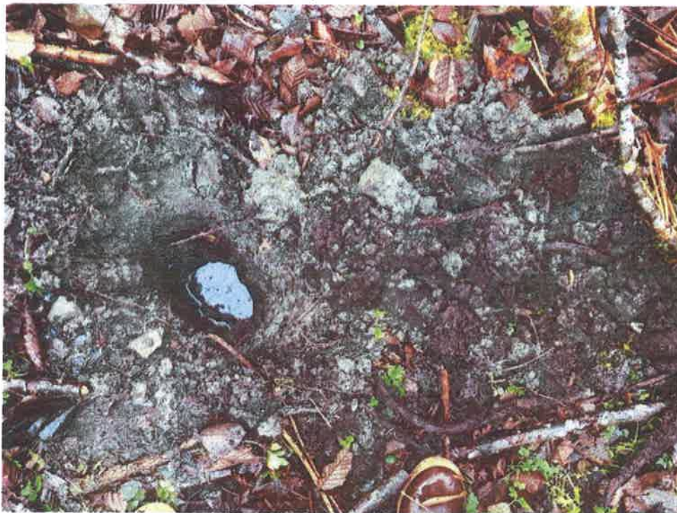
Photo 5 – Eroded fill material with silts and gravels over native organic soils at the toe of the fill pad.
