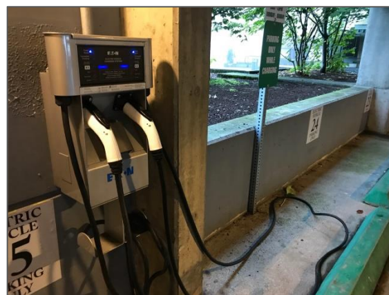
Marine Parking Garage EV Charging Station
