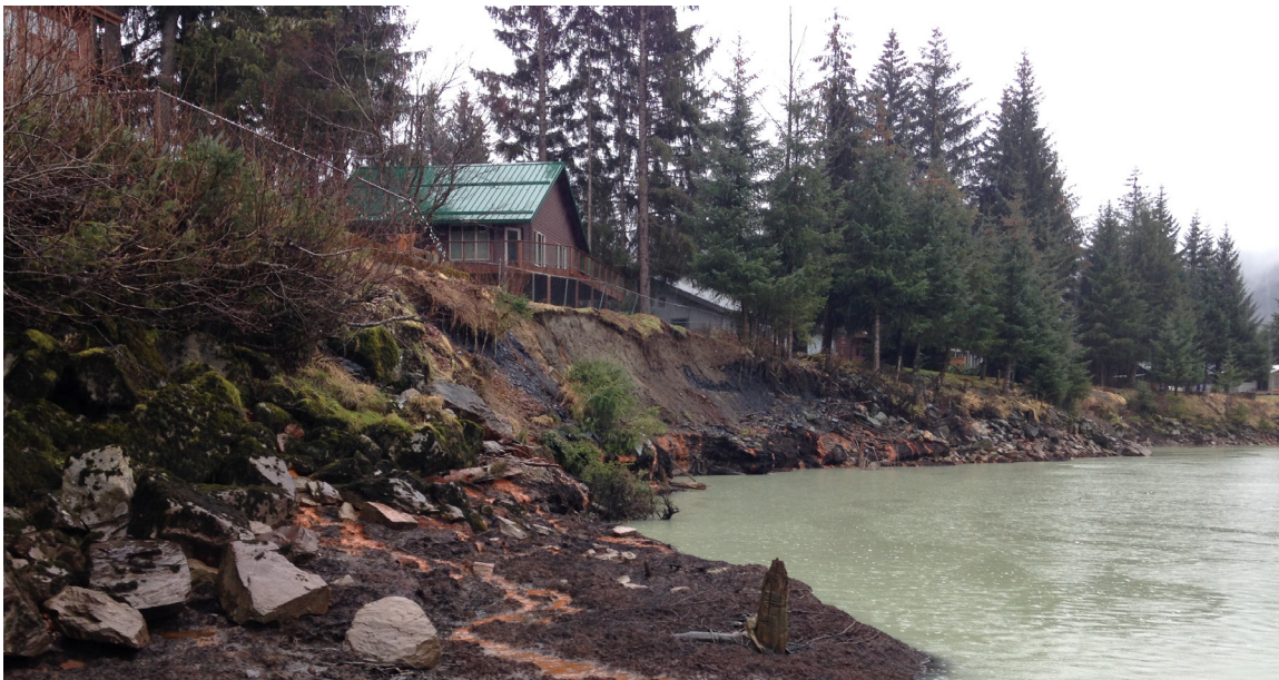
Figure 4: Streambank erosion of the Meander Way bend of the Mendenhall River, March 2015
