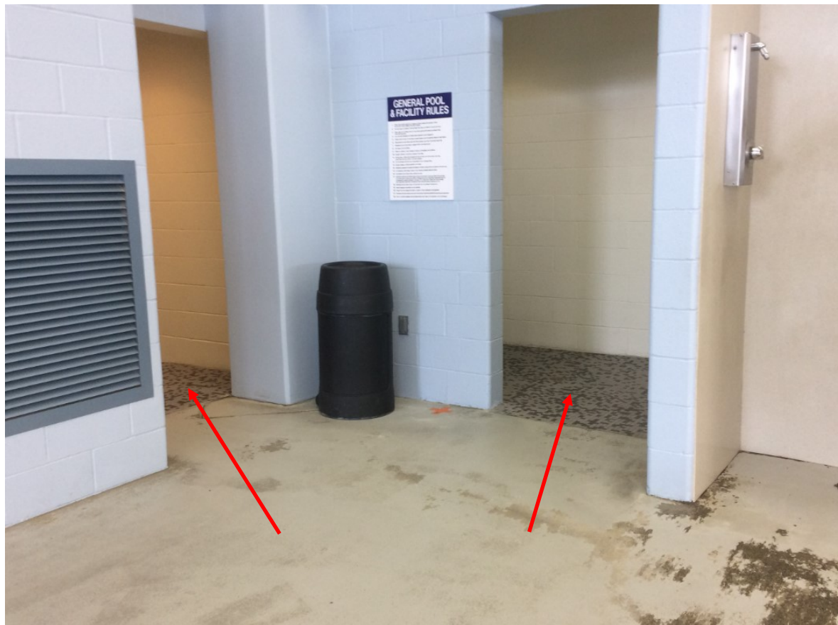
TILE AT LOCKER ROOM ENTRIES TO REMAIN WITH TRANSITION STRIPS ONTO NEW LIFEFLOOR
