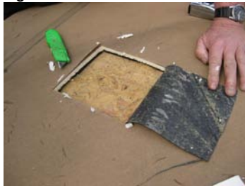
PCV Roof Membrane w/ 1/2" Rigid Insul. EPDM folded back exposing OSB below
