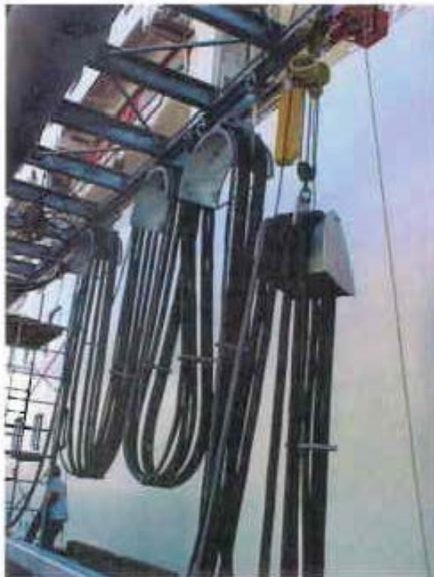
Figure 3 - Shore tie Cable Festoon
