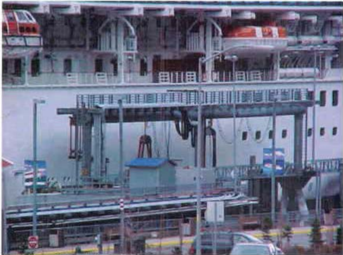
Figure 1 - South Franklin Dock Shore Power
