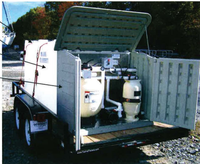
Plastic enclosure for filters, pump, and controls.
