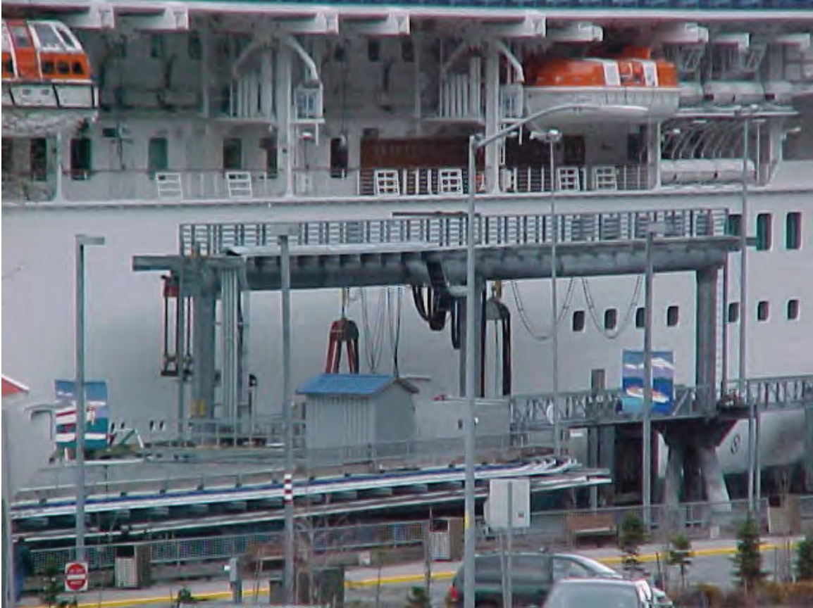
Figure 1 - South Franklin Dock Shore Power
