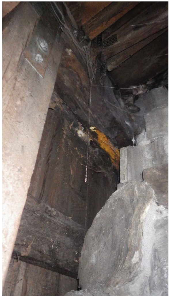
Deteriorated wall framing behind chimney
