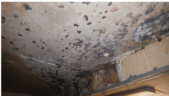
Ceiling damage in mechanical room
