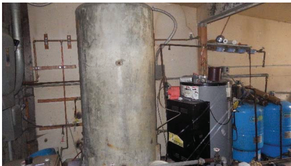
Mechanical room equipment
