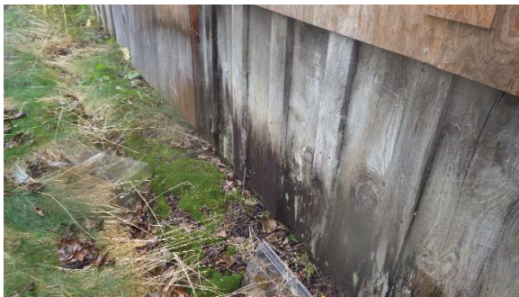
Moisture damage under windows
