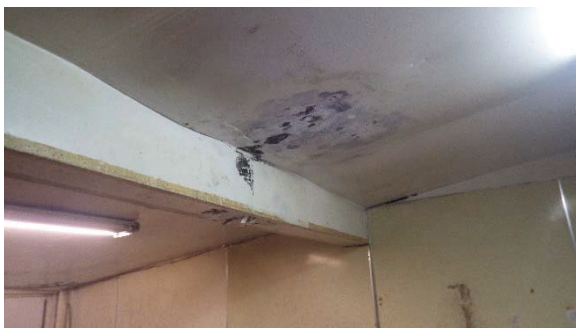
Damaged ceiling in kitchen area
