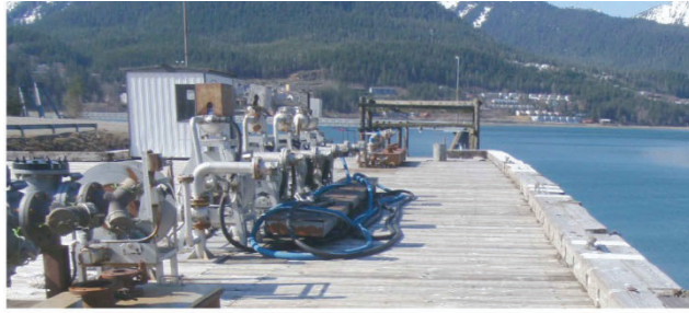
EXISTING FUEL HEADERS
