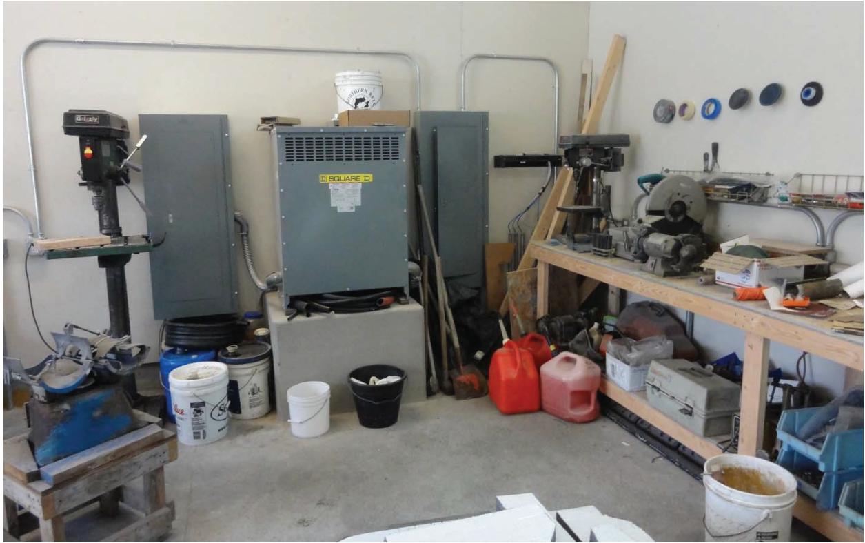
PHOTO 3 - INTERIOR SHOP BUILDING SHOWING ELECTRICAL SYSTEM (051518_2548)
