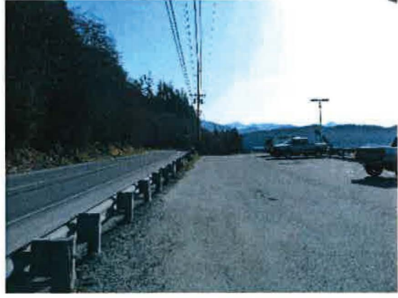
ENCROACHING PARKING AND GLACIER HIGHWAY FRONTAGE 040612_0891
