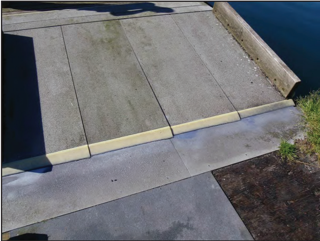
Transition plate assembly – worn UHMW nosing pieces.
