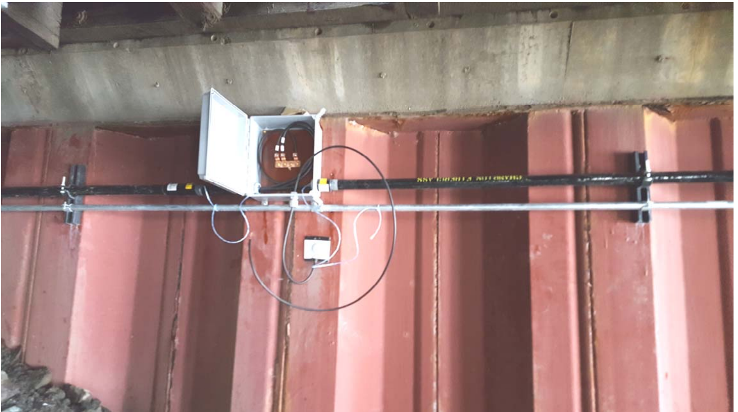
Photo 2: West Wall Bond Box
