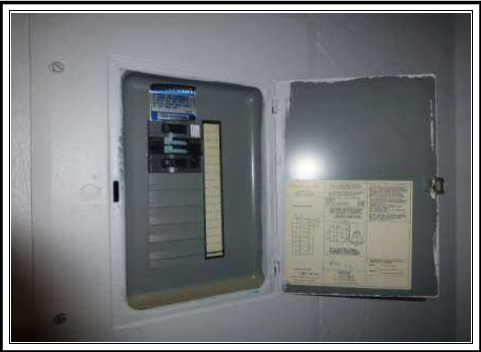
Electrical Panel - Sylvania
