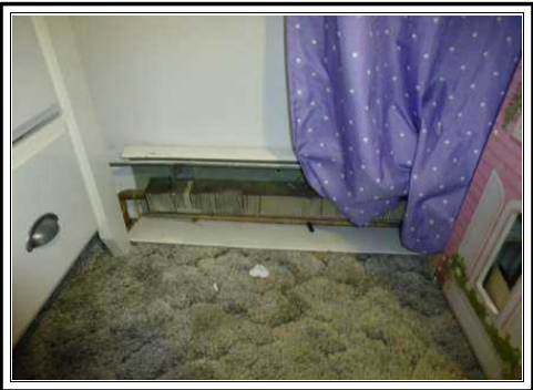
Baseboard Missing Cover
