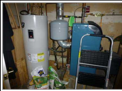
Water Heater and Boiler
