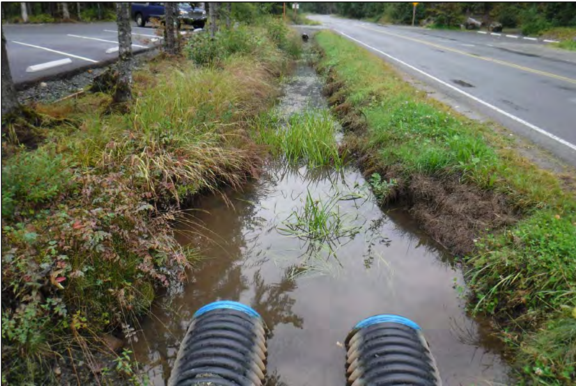
Figure 5.—Plastic culverts under Skater's Cabin parking lot driveways.
