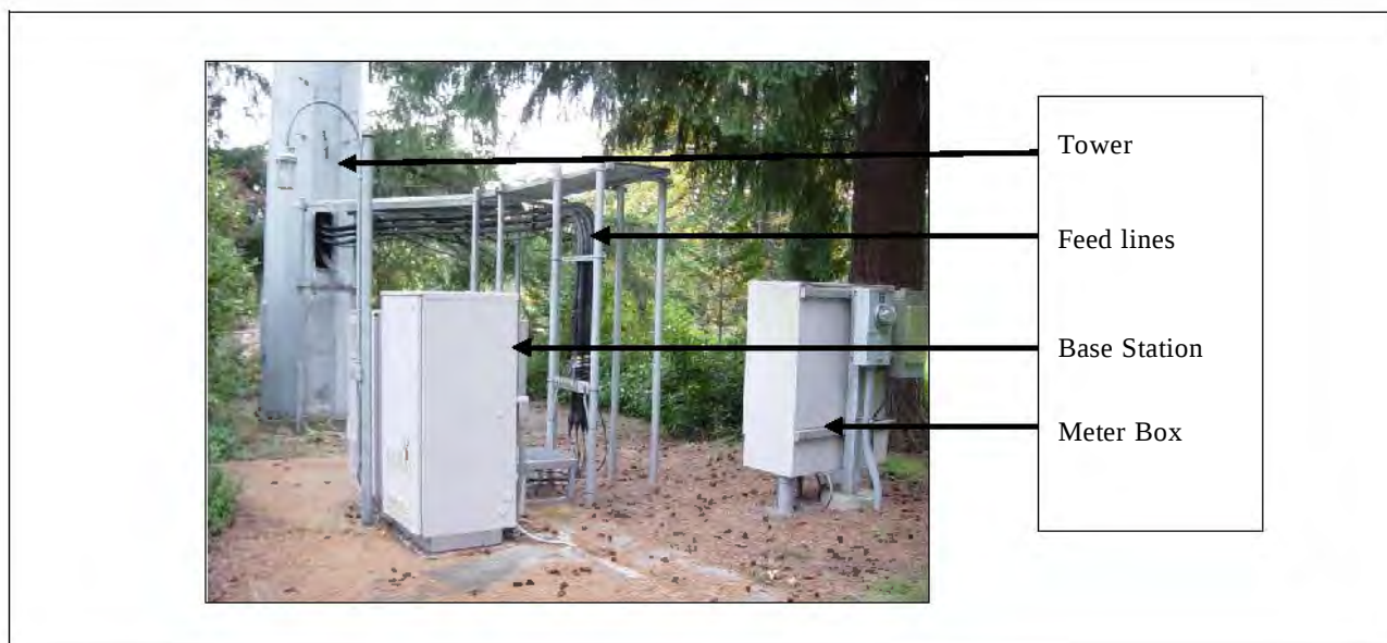
Figure 1: Example of 1900 MHz Wireless Infrastructure Ground Equipment
