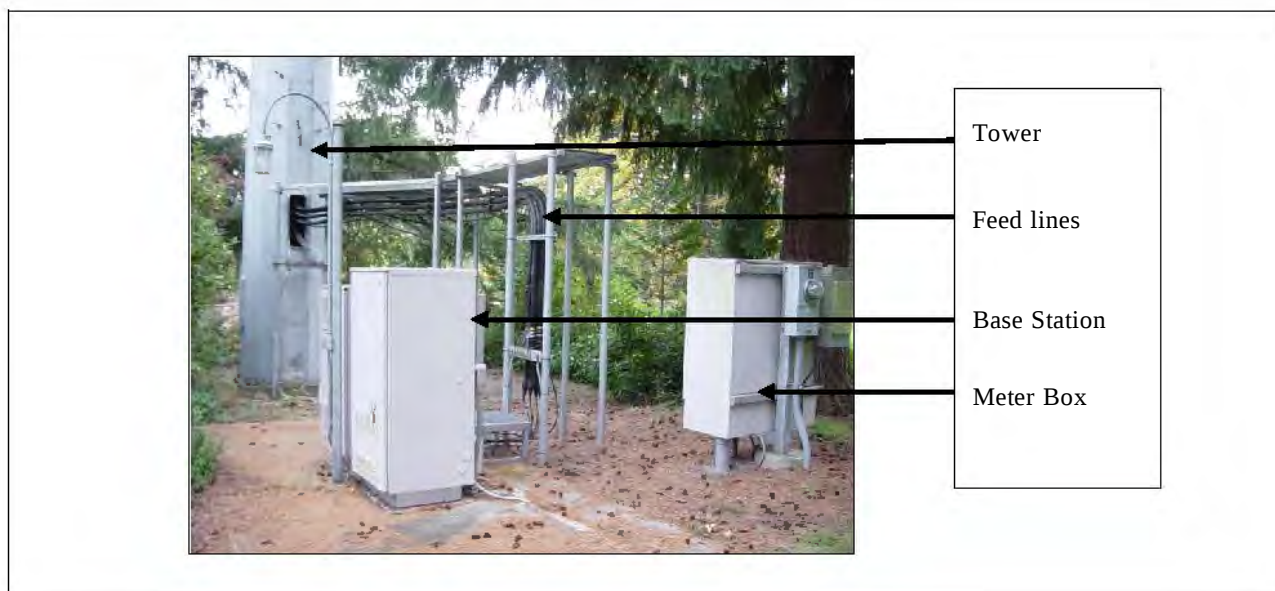
Figure 1: Example of 1900 MHz Wireless Infrastructure Ground Equipment
