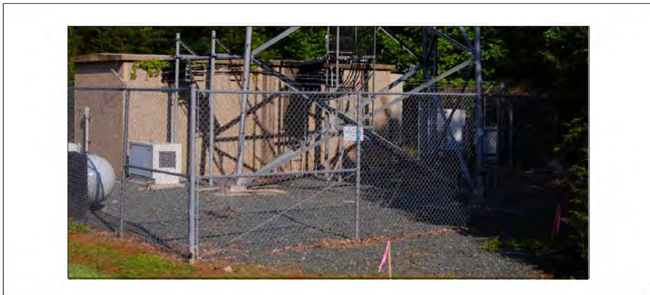
Figure 2: Example of 800 MHz Base Station
