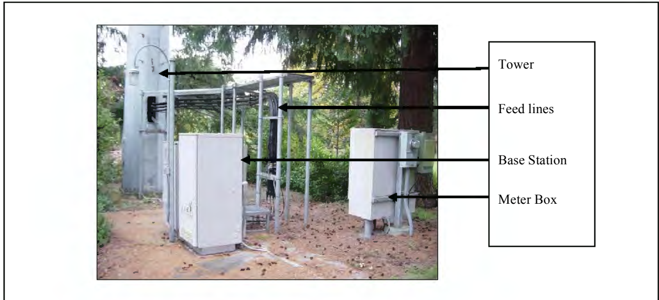
Figure 1: Example of 1900 MHz Wireless Infrastructure Ground Equipment
