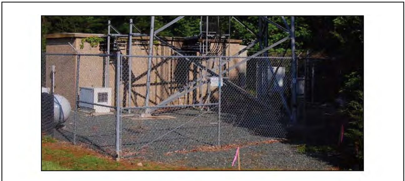
Figure 2: Example of 800 MHz Base Station
