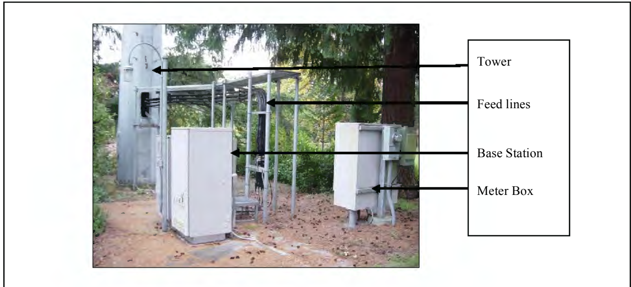
Figure 1: Example of 1900 MHz Wireless Infrastructure Ground Equipment
