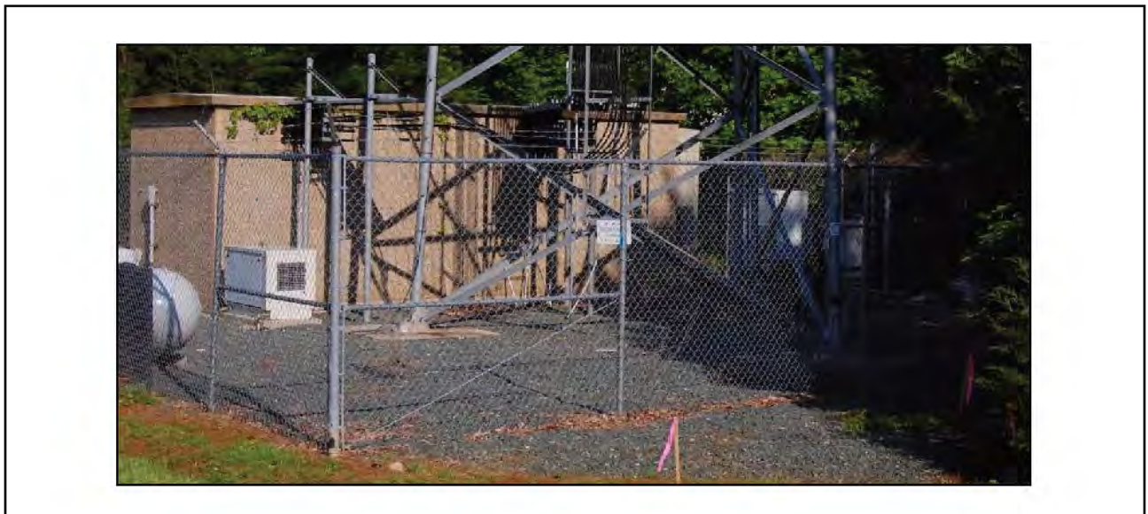
Figure 2: Example of 800 MHz Base Station
