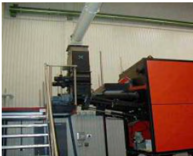
FIGURE 4 BioCon-ERS Incinerator Furnace
