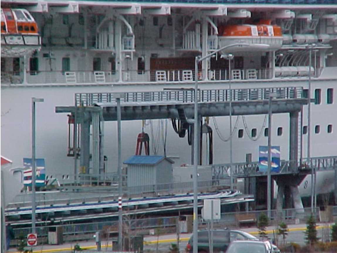
Figure 1 - South Franklin Dock Shore Power
