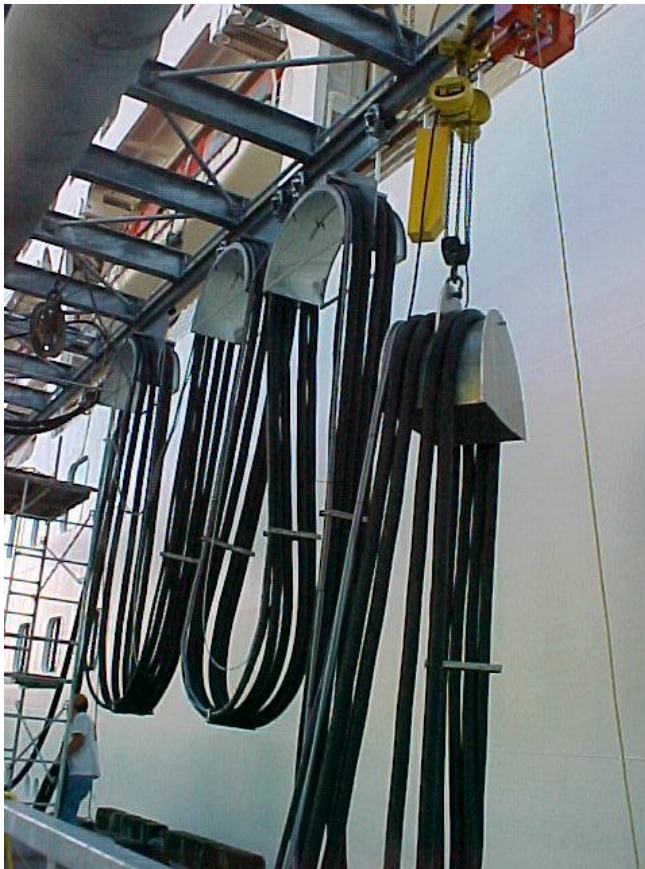
Figure 3 - Shore tie Cable Festoon
