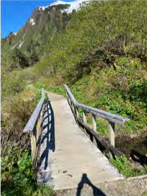
Broken bridge on Perseverance Trail (May 2022)
