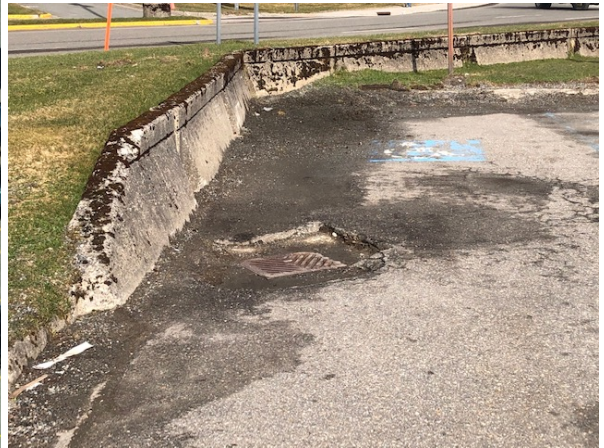
Long term parking lot failing vault
