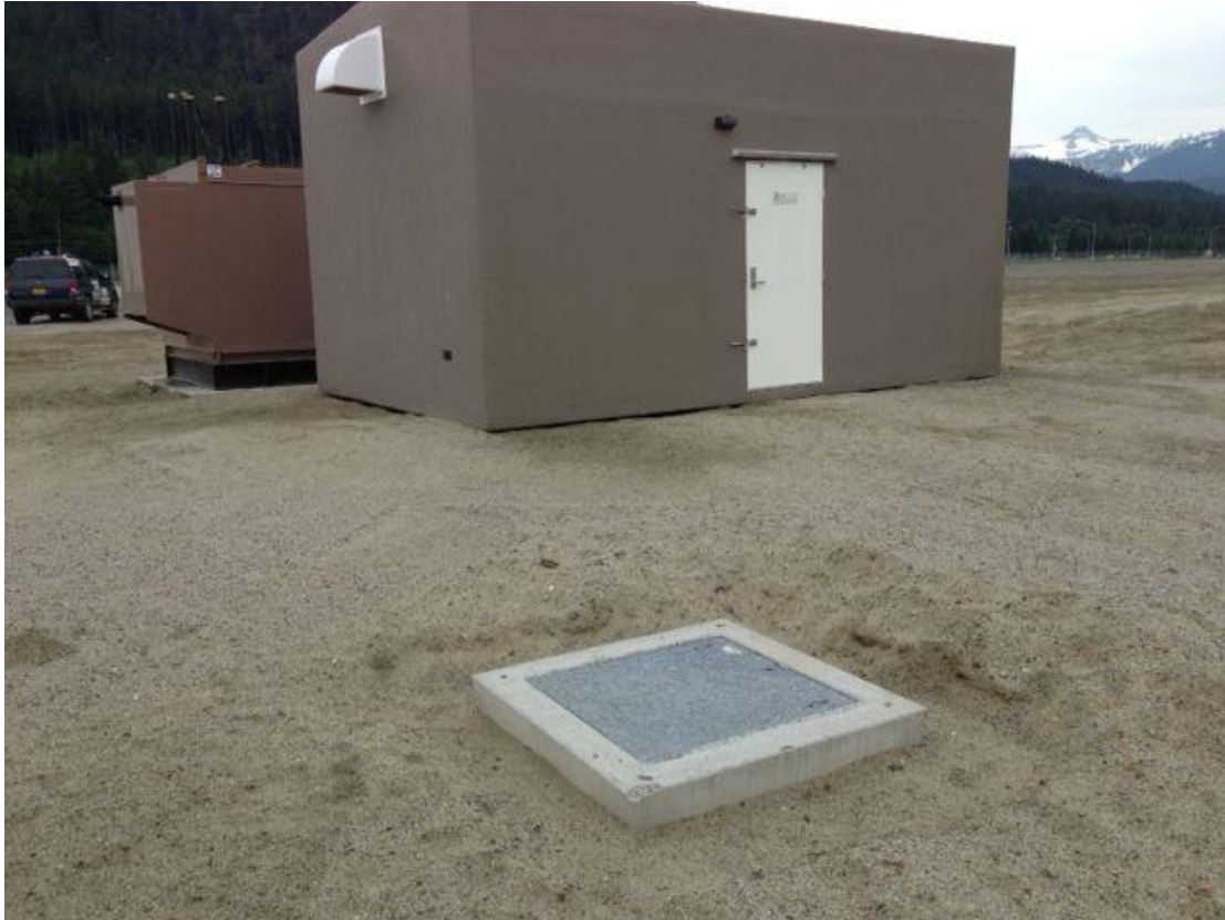
New Regulator Vault and Emergency Generator
