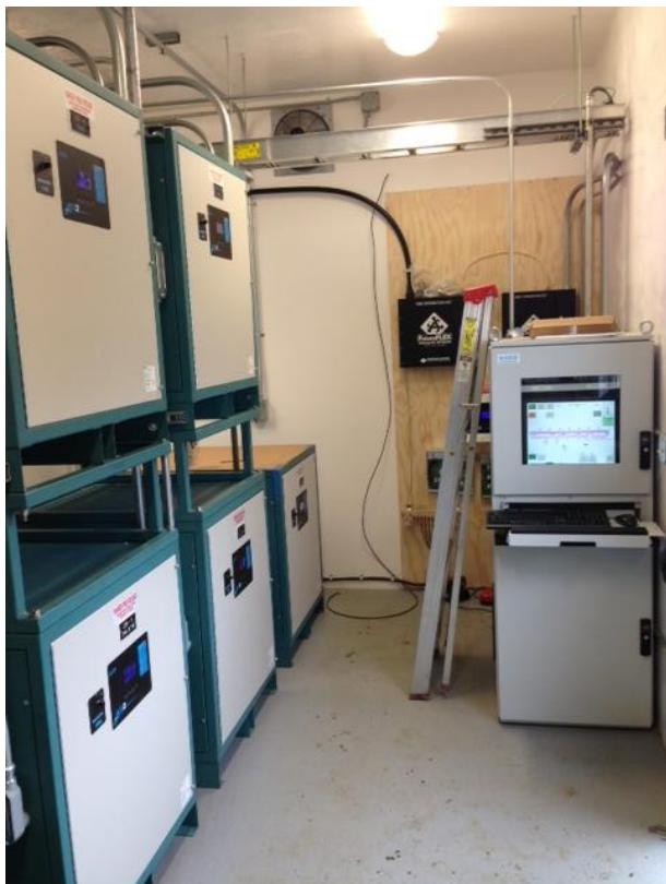
New Regulator Equipment and Lighting Controls
