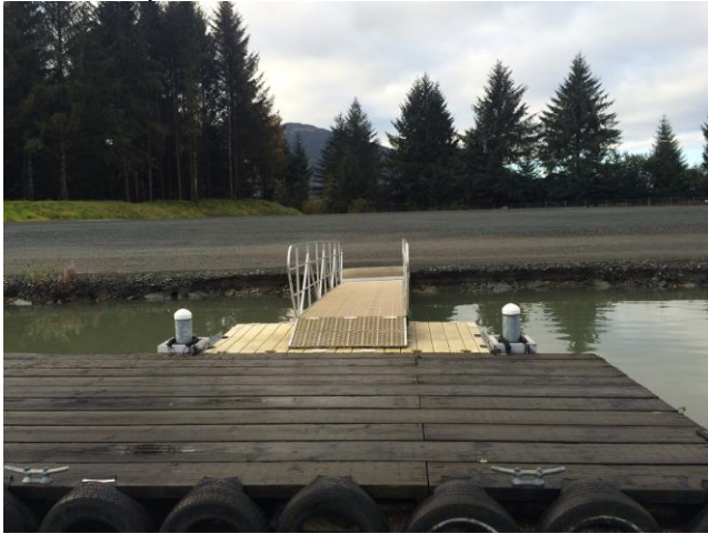
Pictures of South Float Pond shore and dock damage
