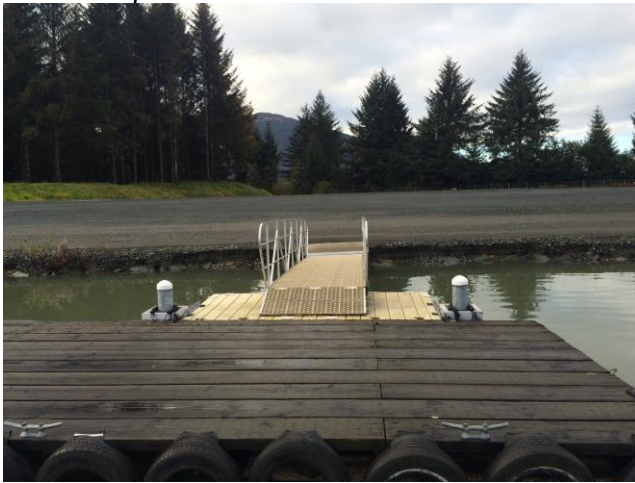
Pictures of South Float Pond shore and dock damage
