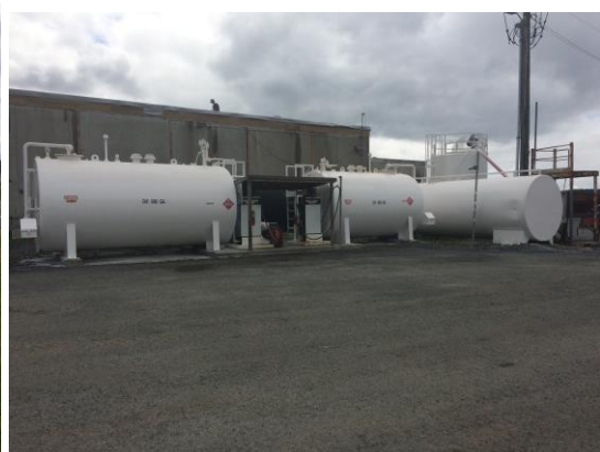
Freshly painted/marked fuel tanks.
