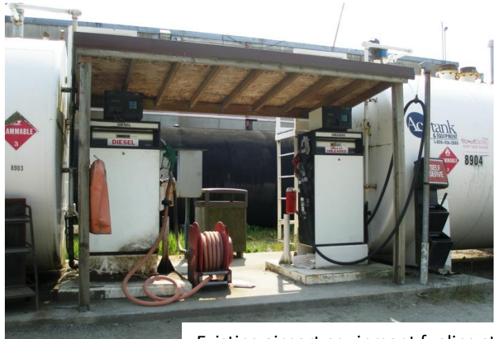
Existing airport equipment fueling station.
