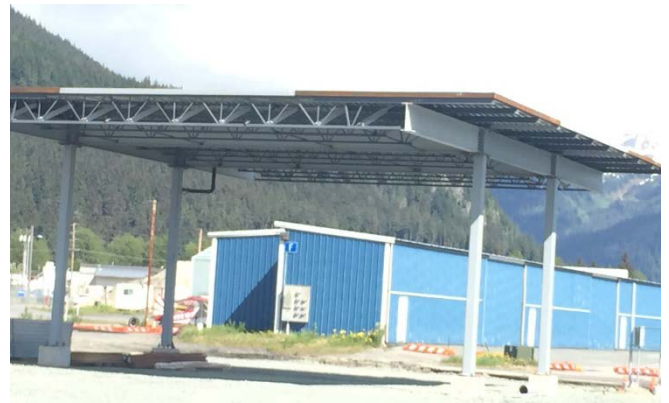
Fueling Station Canopy
