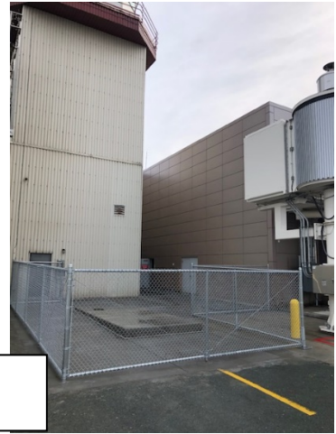
Utility alcove ready for service equipment.
