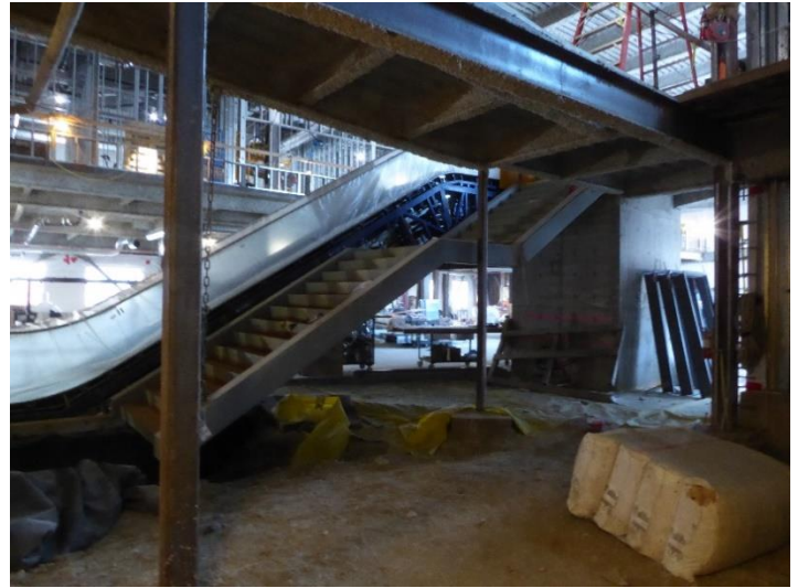
Escalator installed adjacent main stairway.
