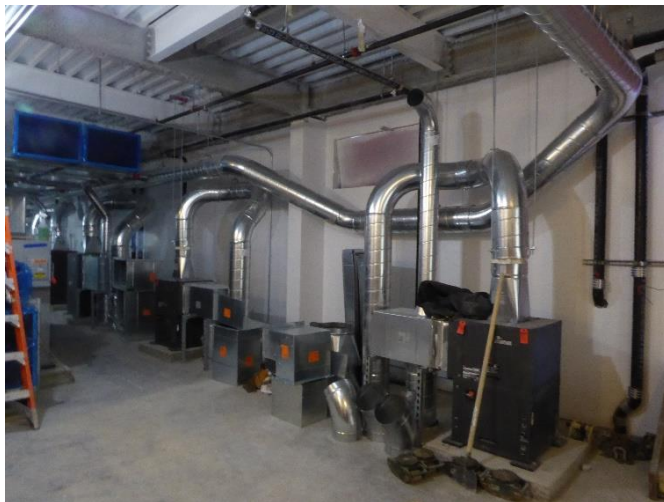
Heat pumps along west wall in penthouse.
