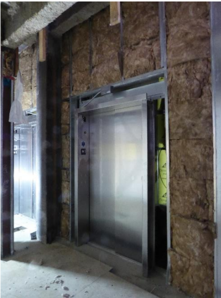
1 st floor elevator entrances.
