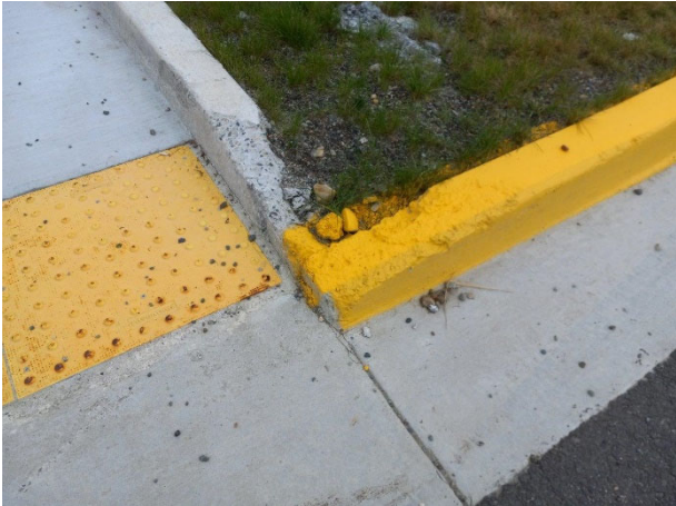
PHOTO 06: Damage at one of the accessible ramps.
