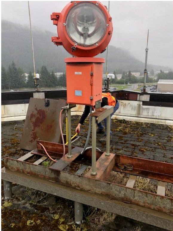
PHOTO 01: Rotating Beacon and Steel Support Assembly
