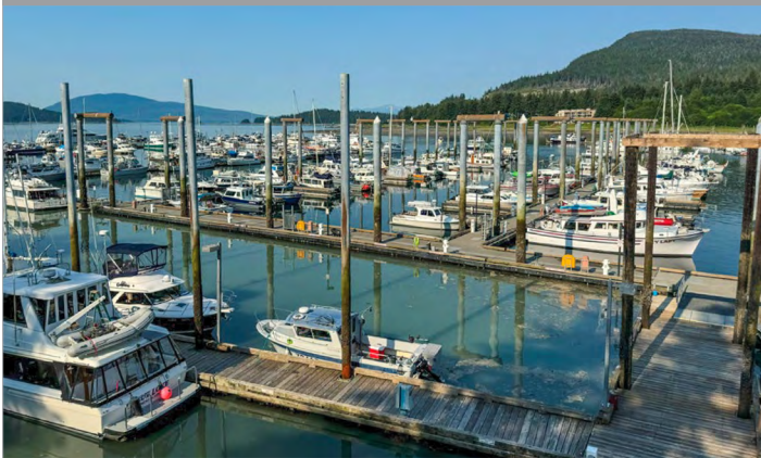
Figure 1: Aging Piles and Floats at Statter Harbor
