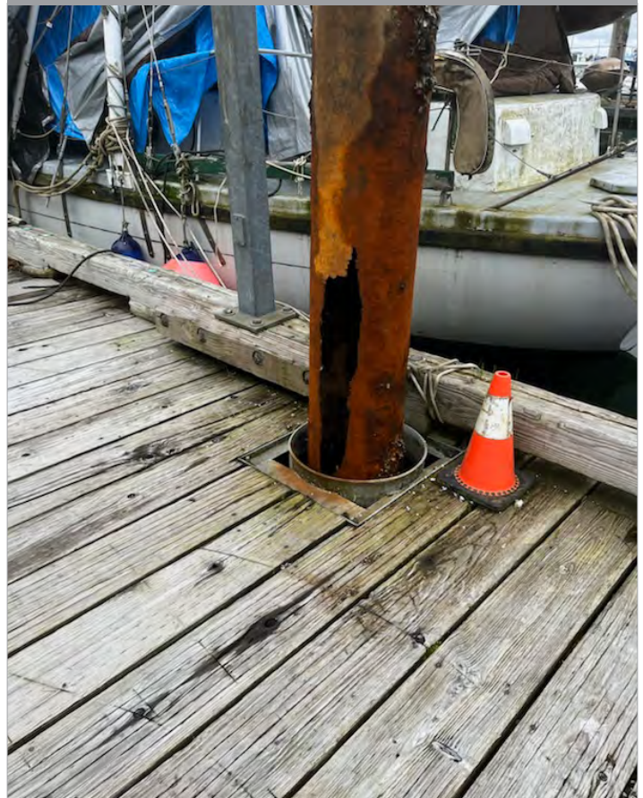
Figure 10: Corroded Steel Pile
