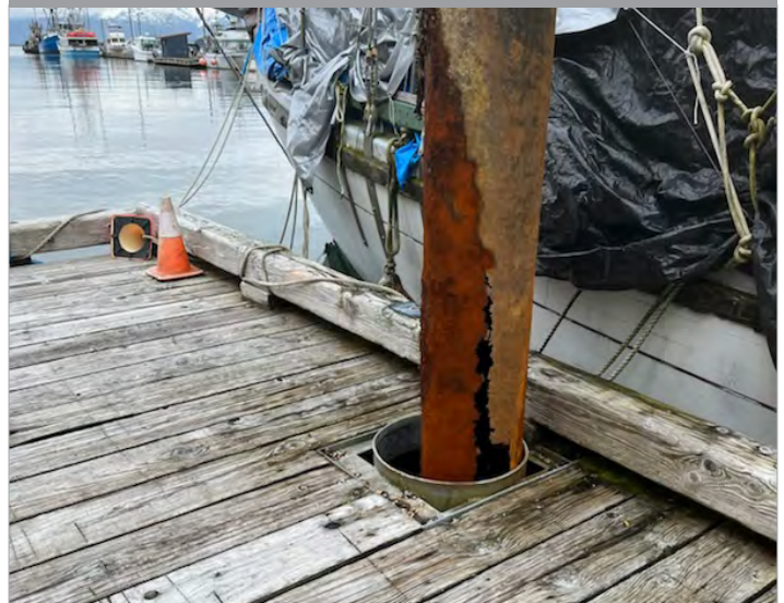
Figure 2: Corroded Steel Pile
