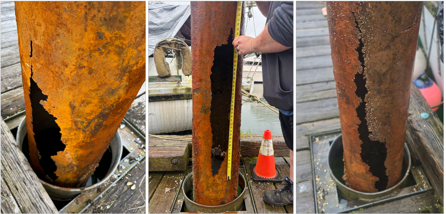
Figure 5: Deteriorated Piles at the East Side of the Harbor
