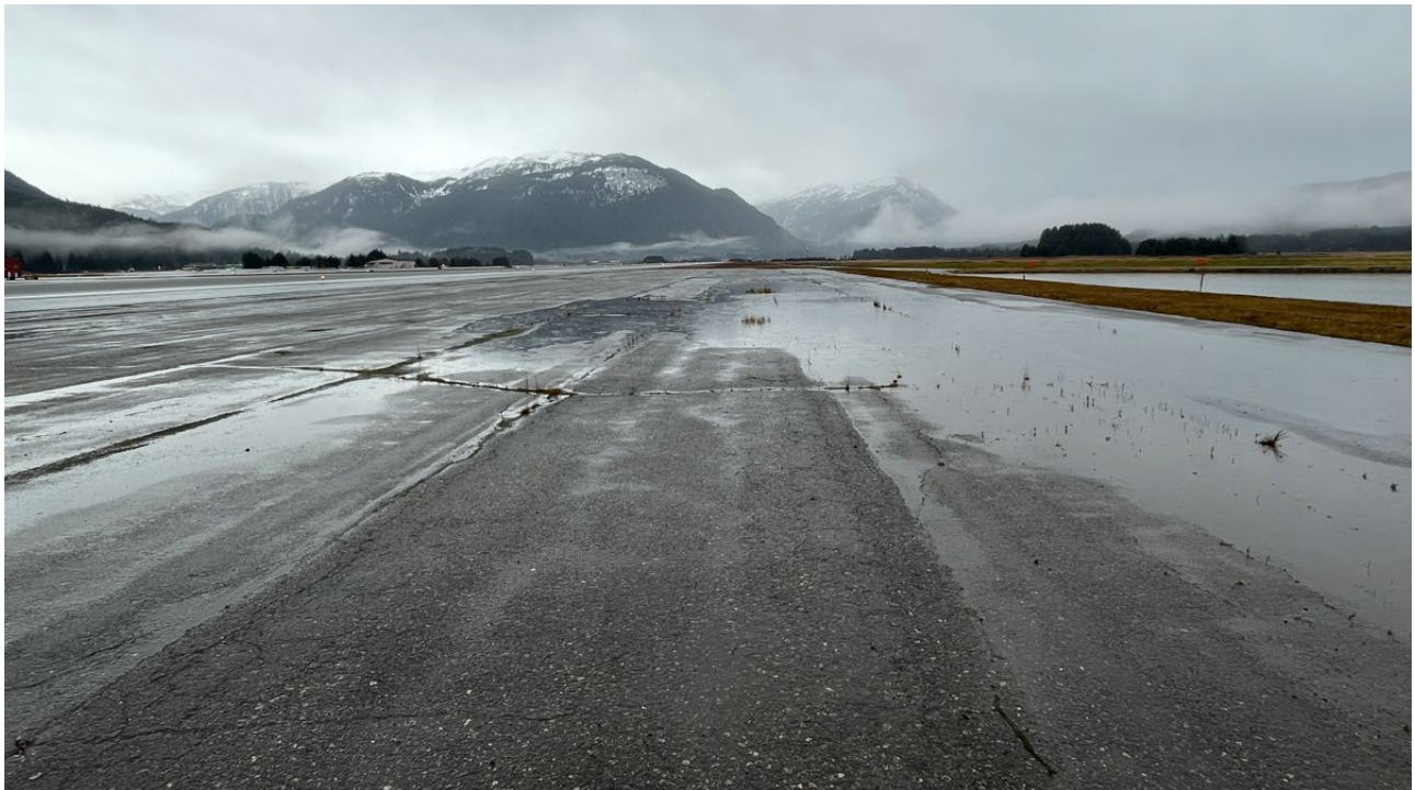
Photo 2: Looking east. Uneven paved surface and ponding along the south edge of the paved surface
