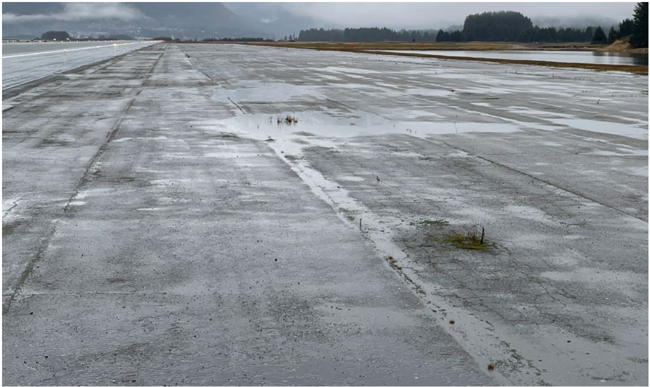
Photo 1: Looking east. Uneven paved surface exhibiting ponding.
