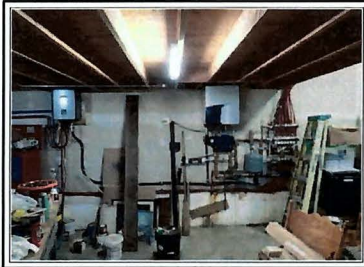
Utilities in Garage
