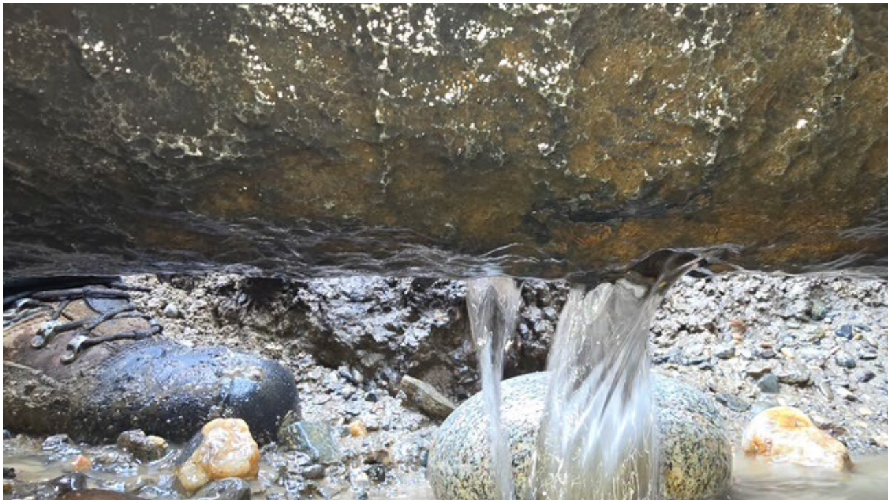
Extreme Pitting and Corrosion of Waterline and Leak
