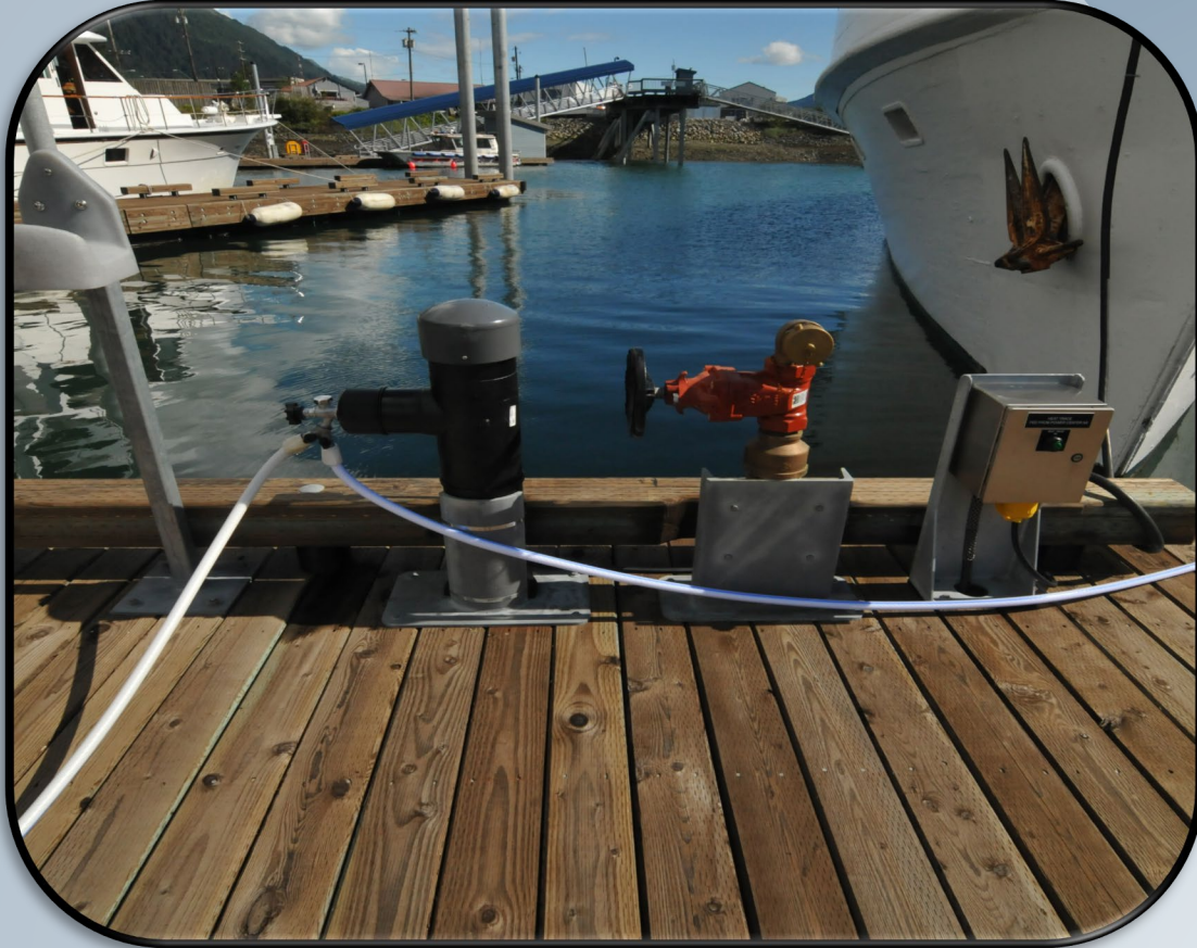
Freeze Protected Water & Fire Suppression Pedestal
