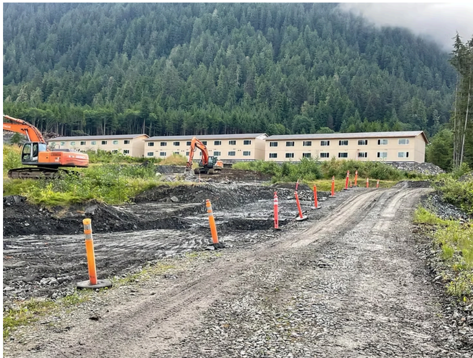
Work at the Chilkat Vista Apartments site on Aug. 2, 2025. (Laurie Craig / Juneau Independent)
