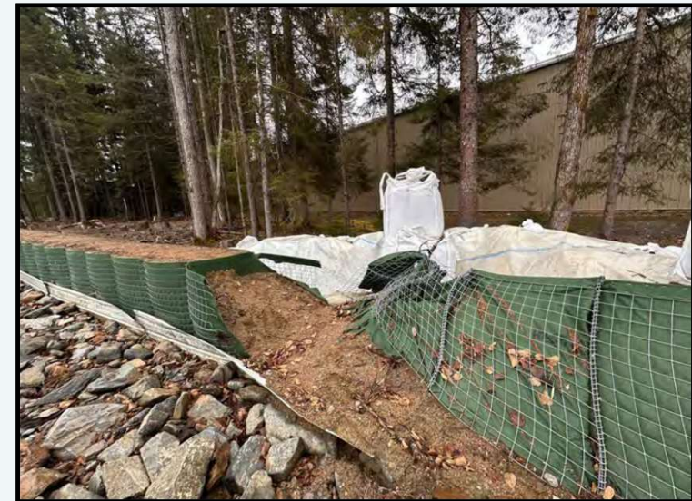
Damaged / breached HESCO barrier from tree impact during turbulent river flow
